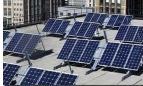
Roof Top Solar PV
