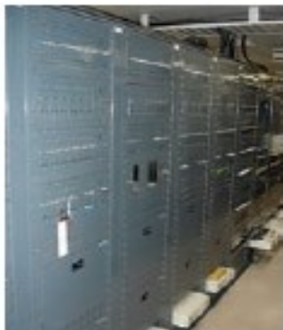
Figure 1 - Equipment bay containing legacy transmitter equipment
